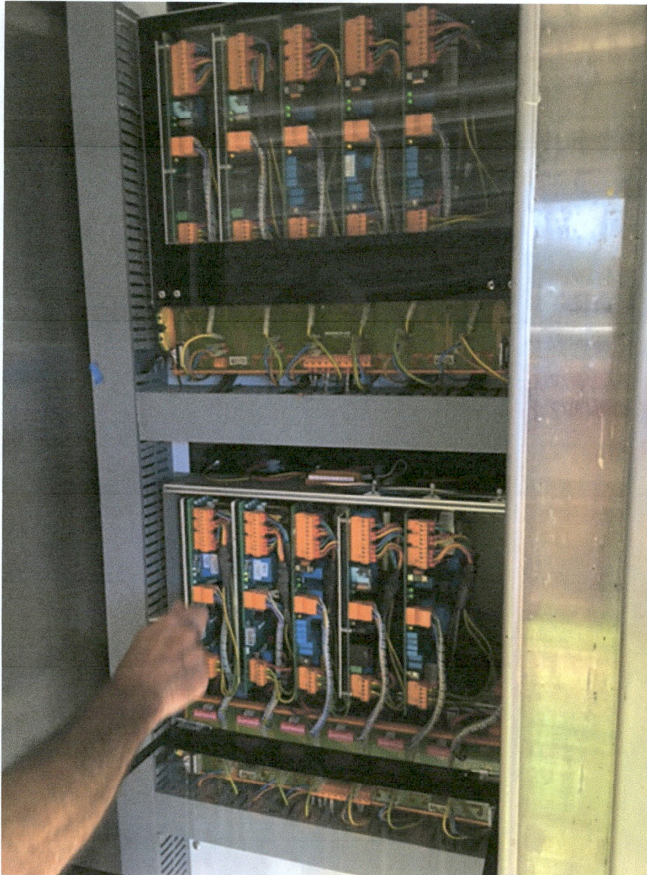
FIGURE 2.4 CONTROL CENTER – BALLAST CABINET
